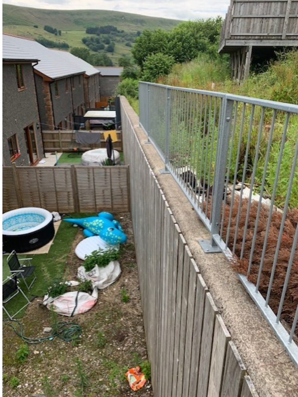
Photograph 13: showing the large retaining wall faced with timber boarding provided to the rear of properties 4-7 Rhys Yr Ysgol
