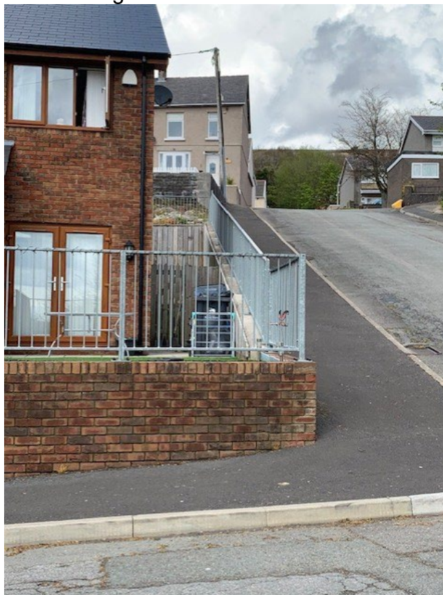
Photograph 14: showing mass concrete retaining wall supporting the highway footway on the sites eastern boundary
